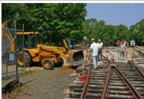
More Ballast Please? Adrian Adkins drops ballast in the area of some new trackage at the museum. (R.A. LaMay Photo)
