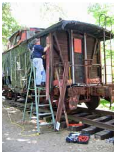
Member William Bouchelle starts to remove the chard lumber in the early restoration stages for the CV 4052 caboose. (Stuart Coleman Photo)
