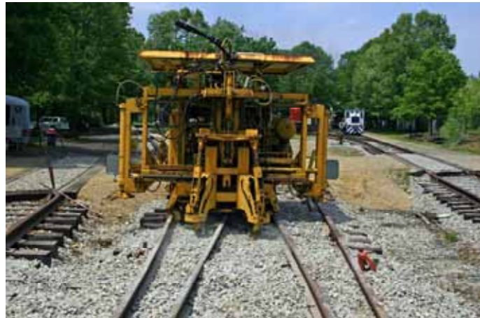
On 5/26/07 this photo shows the museum's RMC McWilliams Spot Tamper working at the 4 track crossing at the eastern end of the museum grounds opposite the Versailles Ticket Shanty. Photo by R. A. LaMay
