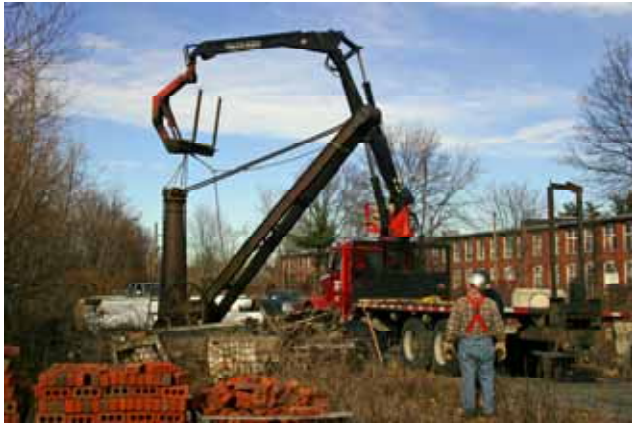
The Farrel Railroad Crane was dismantled and moved to the museum on 1/3/07. Shown here members of the museum with the help of Ken Sigfridson and Fran Minarik prepare the crane to be taken down at Middletown, CT. (R.A. LaMay Photo)
