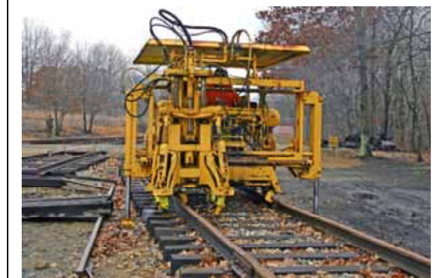
The museum's RMC McWilliams Spot Tamper works along a new section rail under the guidance of Rich Cizik. After a long period of repairs and major part replacement the tamper worked successfully one tie at a time on 1/13/07. (R.A. LaMay Photo)
