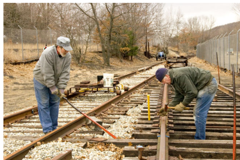
A sure sign of spring. Track work is once again under full swing. Shown here Mark Granville and Art Hall, Jr. work on the #8 switch that will eventually bring rail to the Columbia Junction Roundhouse and Turntable Bridge. (Photo by R. A. LaMay)
