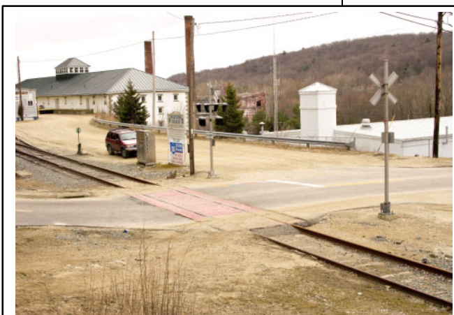
Progress can be seen at the P&W's Rte 97 crossing in Baltic, CT. Note the road plate was installed, the control box, the cross bucks, and the signals on one of the poles. 3/25/06 (R.A. LaMay Photo)
