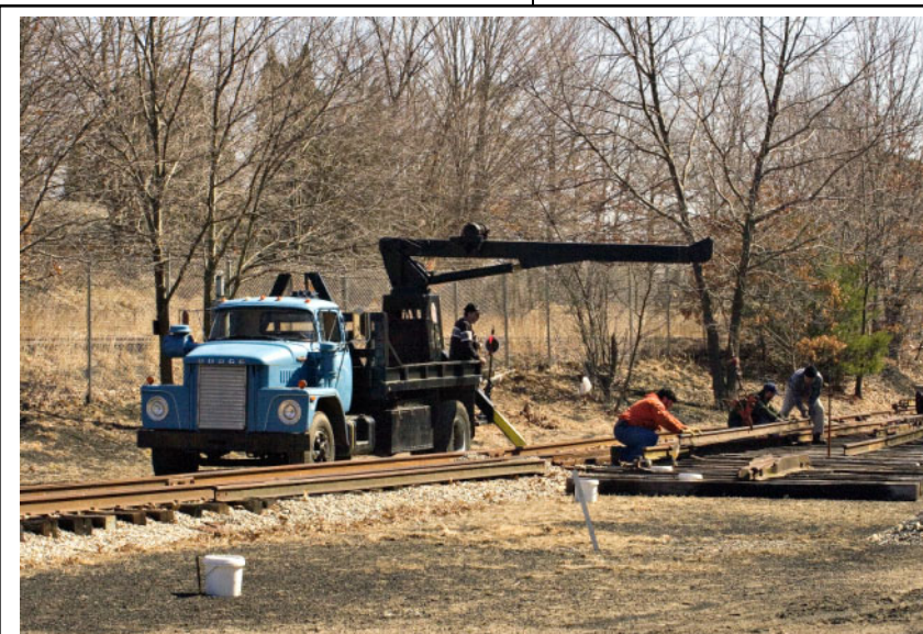
The museum's ex Penn Central boom truck helps members move rail while working on the #8 switch. (Photo by R. A. LaMay)
