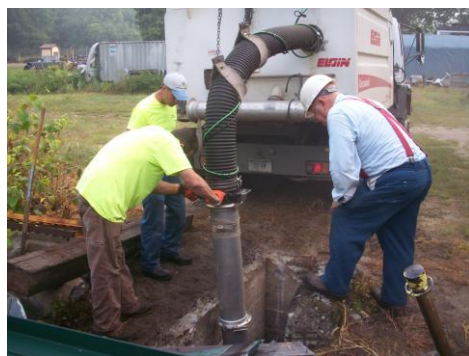
Cliff Lund arranged to have the Willimantic Public Works Dept. catch basin cleaning vacuum truck suck all the small debris out of the concrete riser to a depth of 10 feet. Shown here is the process taking place. (Bob Hassett Photo)
