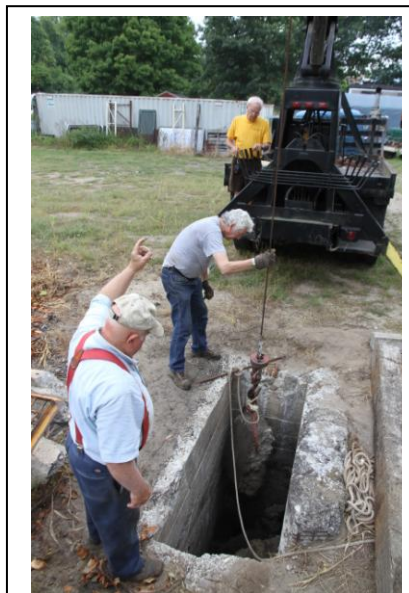
With Dick Arnold operating boom truck, Adrian Atkins giving signals, Art Hall Jr. guides up a large piece of concrete being hauled up out of the cistern. (Robert A. LaMay Photo)
