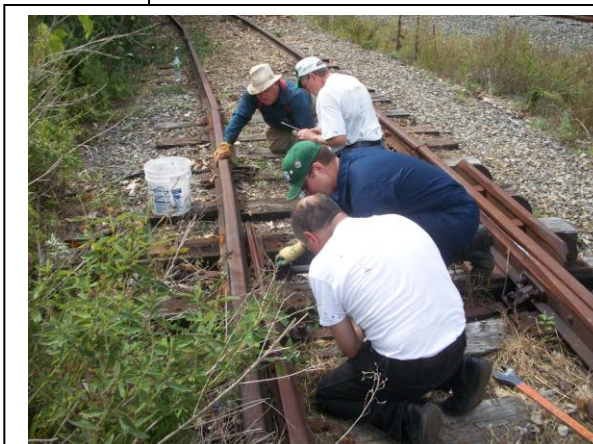
This photo shows Adrian Atkins, Rolf Johnson, Andrew Porter, and Dan Ditullio preparing to remove the switch points along with rail at Dayville, CT. (Cliff Lund Photo)
