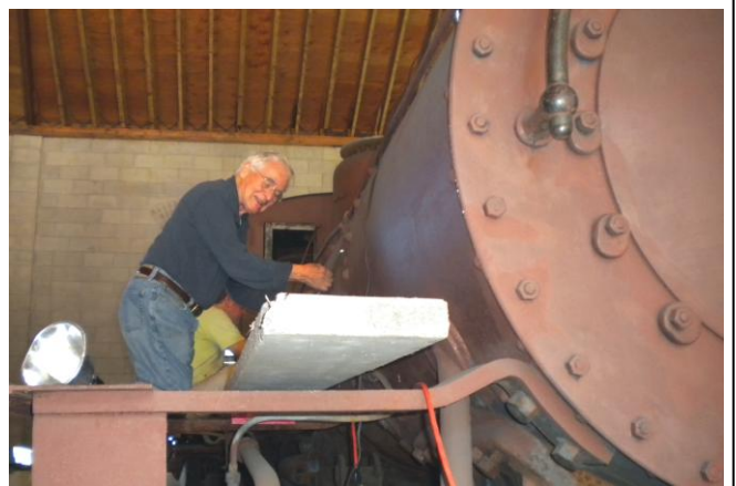
The mapping of the boiler on Steam Locomotive Number 10 has begun. Shown here owner Joe Pagano works on the boiler. Behind him Bill Voorvaart can be see assisting Joe. Photo by Jean Lambert)
