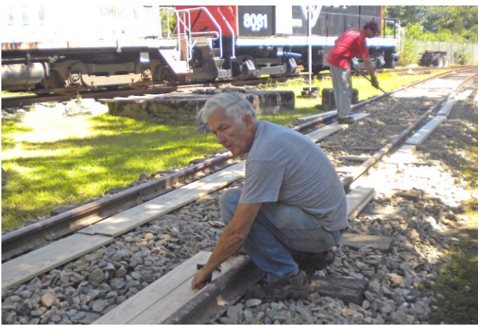
Art Hall, Jr in the foreground and Andy Fischer in the background work on the new passing siding being constructed at the museum. (Jean Lambert Photo)
