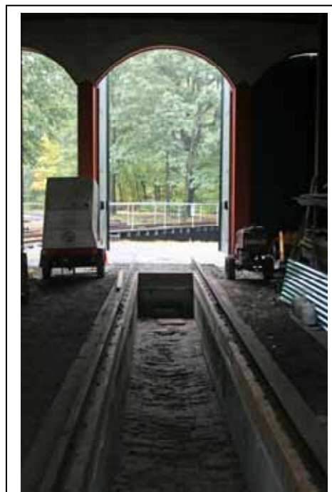
This photo taken 9/27/08 shows the latest progress on Pit no.3, looking toward turntable bridge – R.A. LaMay Photo
