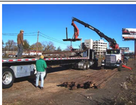
Fred Minarik with Ken Sigfriedson's crane truck loads rail onto Bob Leach's RCW contracting trailer. Evan Sigfriedson and Howard Raphaelson assist with the loading. (Adrian Atkins Photo)
