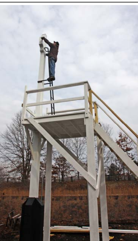
Rolf Johnson makes some adjustments on the Gallows Signal currently under construction at the museum. (Robert A. LaMay Photo)
