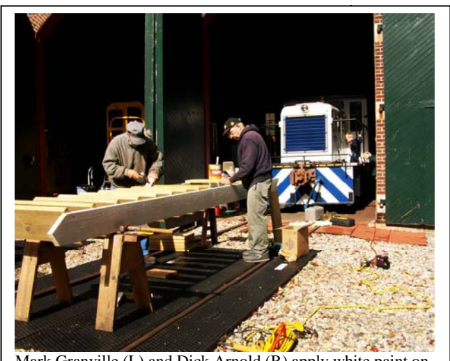
Mark Granville (L) and Dick Arnold (R) apply white paint on Gallows Signal stairs. (Jean Lambert Photo)
