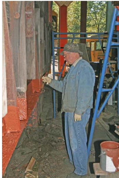
Member Bill Bouchelle applies the protective coat on some recent steel work done during the restoration of the CV 4052 caboose. (Robert A. LaMay photo)
