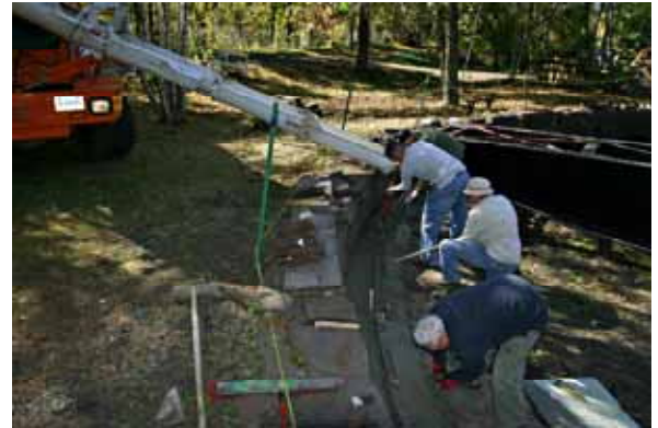
History took another big step on Oct. 16, 2007 when a Builder's Concrete truck started pouring concrete for the ring rail pad in the turntable pit. Members, Dick Arnold, Rolf Johnson, Bob Hassett, Adrian Adkins, Adam Bycholski, and Carol Stanich were on hand to spread and form the concrete into a ring rail pad. (Robert A. LaMay Photo)
