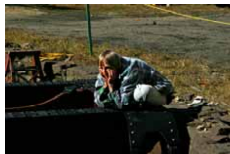
Bridge Boss Carol Stanich, observes the installation of the ring rail at the other end of the turntable bridge. (Robert A. LaMay Photo)
