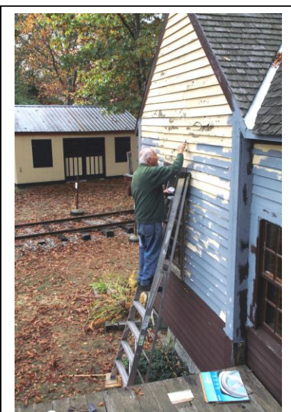
Walt Dumas scrapes off old paint and replaces the necessary wood before a new coat of paint can be added to the Chaplin Station. (Robert A. LaMay Photo)
