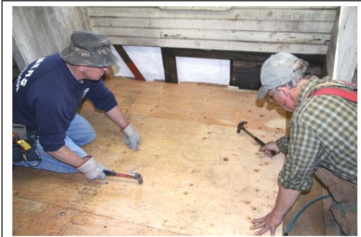
William Bouchelle on left and Duke York on right pound in the final nails of the sub flooring inside the Central Vermont Center Cupola Caboose number 4052. (Robert A. LaMay Photo)
