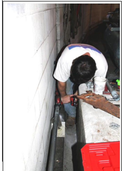
Bill Voorvaart works on the Compressed Air Distribution System inside the roundhouse. (Robert A. LaMay Photo)
