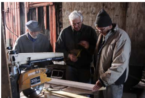
Left to right, Mark Granville, Art Hall, Jr., and Dick Arnold carefully measure the railing supports which will go on the upper platform of the Gallows Signal. (Robert A. LaMay Photo)
