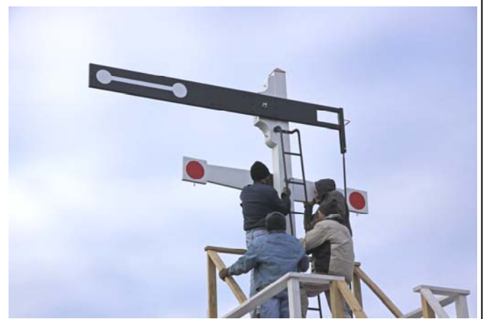
Andy Fischer (upper left) tightens the lower signal board on the Gallows Signal. Both signal boards were put in place on Dec. 4, 2010. Assisting were Bill Bouchelle (lower left), Art Hall, Jr. (upper right), and Dick Arnold, Gallows Signal Design Mgr (lower right). (Robert A. LaMay Photo)
