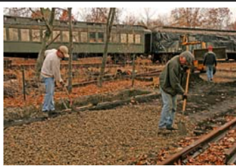
Andy Fischer (L) and Art Hall, Jr. smooth out ballast which will help with drainage near the ash-pit track. (Robert A. LaMay)
