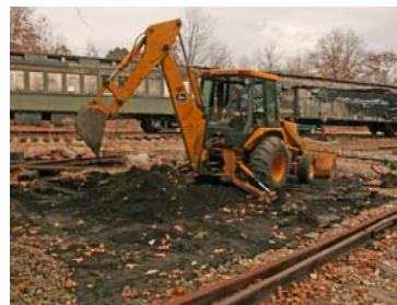
Adrian Atkins continues to grade for the Ash-pit and caboose track switch. (Robert A. LaMay Photo)
