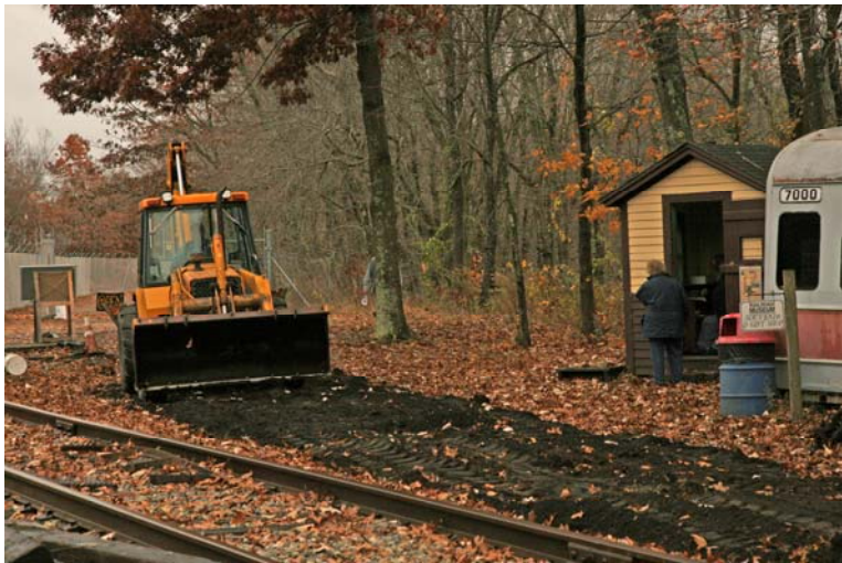
Adrian Atkins smooths the new fill along the roadway in front of museum's gift shop and admission center. (Robert A. LaMay Photo)
