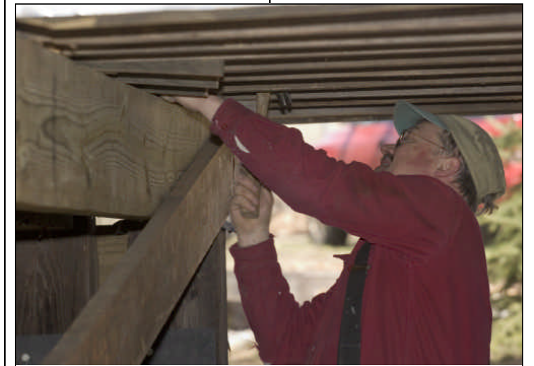
Duke York works under the Groton Freight House replacing some rotted timbers. Thomas J. Nanos photo
