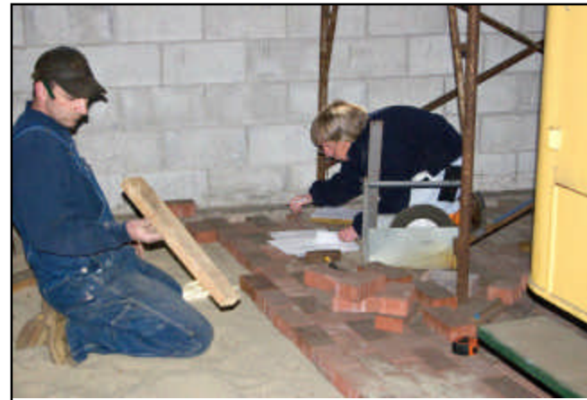
Working on laying engraved pavers in the Roundhouse floor R.A. LaMay photo
