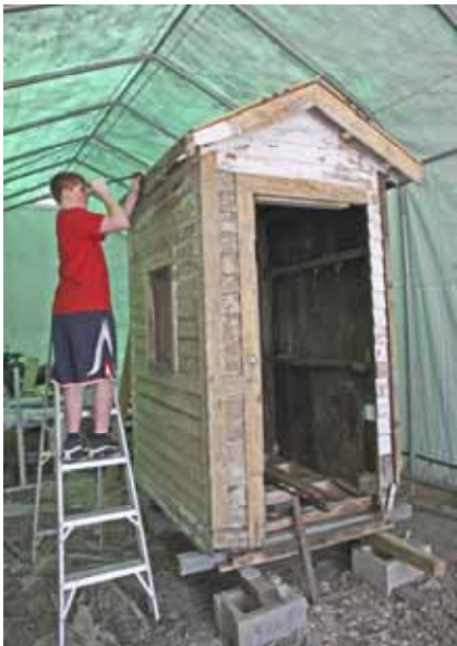
Owen Pender works on his Eale Scout project. He is shown here stripping the Chaplin Operators Shanty. The restored shanty should be back at the museum During the middle of May 2010. (Robert A. LaMay Photo)
