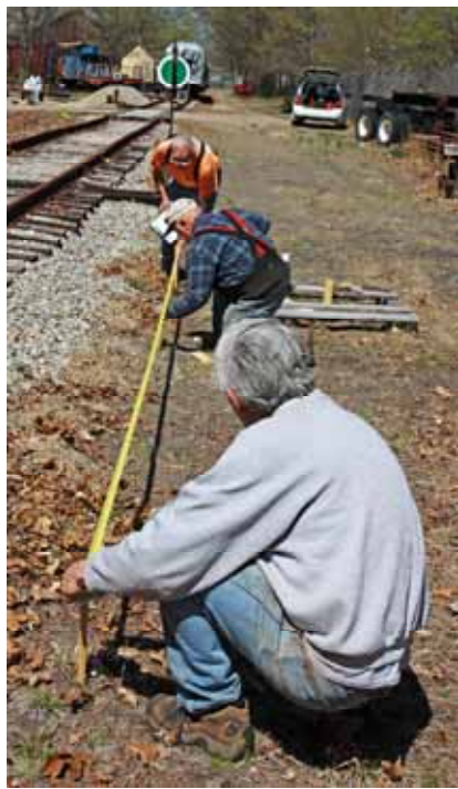
Measurements take place for the re-building of the Gallows Signal that once stood at Bridge St. Dick Arnold (top) takes a reading from the tape. Adrian Adkins places stake as a marker, while Art Hall Jr. holds the other end of the tape. (Robert A. LaMay Photo)
