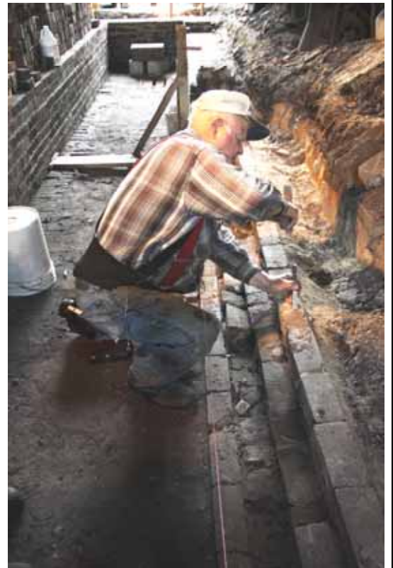
Adrian Adkins chips away at old mortar from the old brick wall that lines Pit NO. 2. Once cleaned new mortar will be put in place. (Robert A. LaMay Photo)
