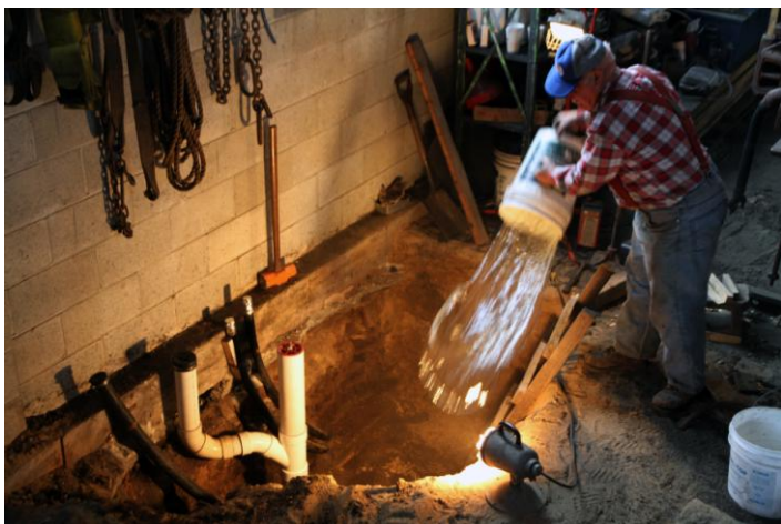
Preparing the roundhouse for water, air, sewage, and electricity takes a lot of preparation. Shown here Adrian Atkins our dirt and sand scientist pours water to assure a flat floor inside the roundhouse. (Robert A. LaMay Photo)
