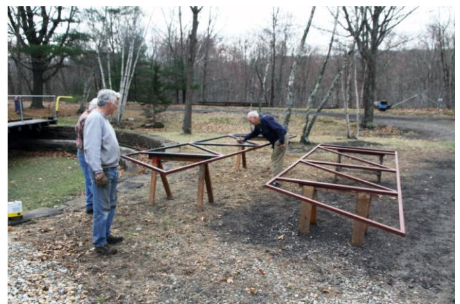
Dick Arnold on the right applies a protective coating to the steel super-structure that will be used when the roundhouse doors are rebuilt. (Robert A. LaMay Photo)
