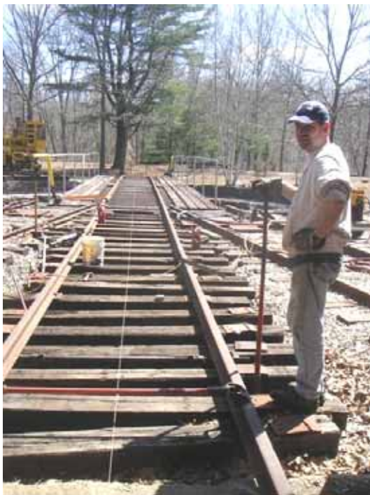
Andy Fischer checks to make sure the alignment string is correct on track number 4 during its restoration. (Robert Hassett Photo)
