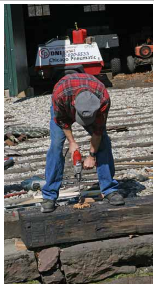
Photo right – Mark Granville drills holes Necessary to hold timbers in place in front Of pit number 2. Once this is done – rail and Ties will be put down – (RA LaMay Photo)
