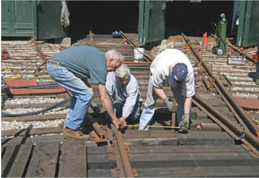
Dick Arnold, Art Hall, Jr. and Andy Fischer mark the necessary places while aligning track 4 during its restoration. Ongoing progress continues on Pit tracks 1 thru 3 to the left. (Robert A. LaMay Photo)
