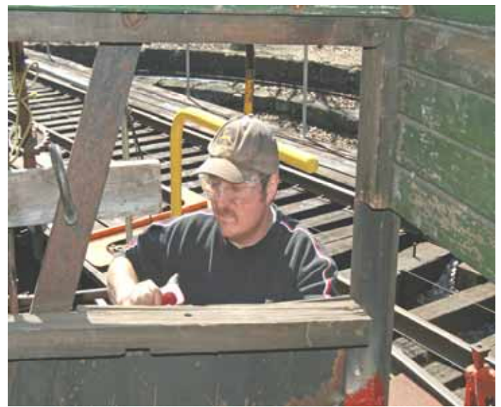
Bill Voorvaart works intently on cutting out the bad areas on the CV 4052 caboose. (Robert A. LaMay Photo)
