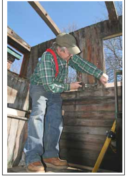
In the photo to the right, Duke York Performs some badly needed restoration In the cupola of the Central Vermont 4052 caboose project. (RA LaMay Photo)
