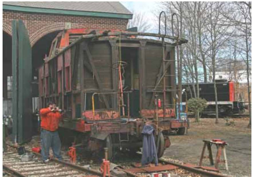
Rich Cizik works on getting some badly rusted bolts during the restoration of the Central Vermont 4052 caboose project. (Robert A. LaMay Photo)
