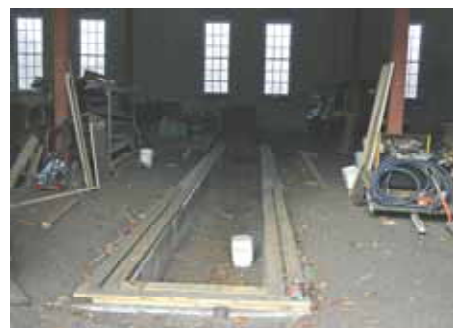
While there is a lot of activity going on around the turntable pit, more work is continuing inside the roundhouse on Pit #4. (Robert A. LaMay Photo)
