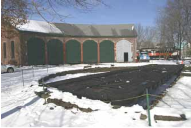
Taken 2/25/08 this shows the progress to date on the turntable. The next step should involve putting the rail down across the bridge. (Robert A. LaMay Photo)
