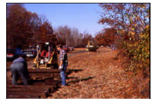
Trackwork along the Air Line. As you can see, there was nothing when we got here. Fall 1994
