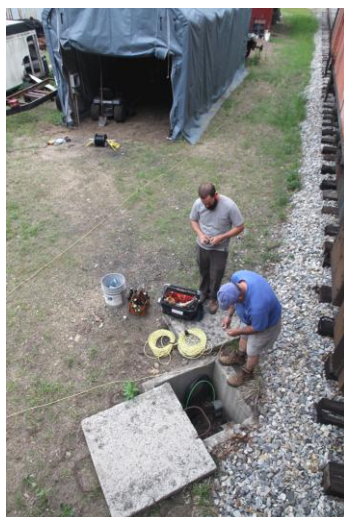
Jim Brennan along with his son Mike installs a new line to the small equipment tent at the museum. (Robert A. LaMay Photo)
