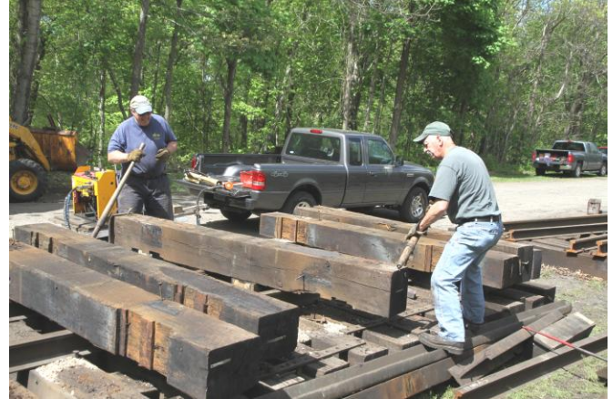
Steve Melady (L) and Gerald Roy are taking apart the track panels received from the Niantic River Railroad Bridge Replacement project. (Robert A. LaMay Photo)
