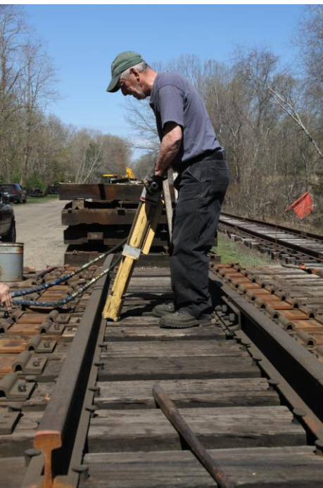
Gerald Roy handles the air powered spike remover as he removes both rail and spikes from the Niantic River Railroad Bridge track panels. (R.A.
