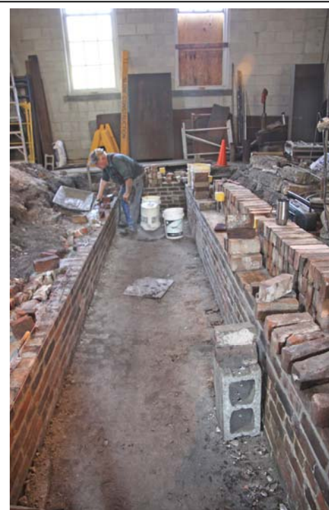
Adrian Atkins continues work on the restoration of Pit no. 2. This turned out to be a major restoration job. (RA LaMay Photo)
