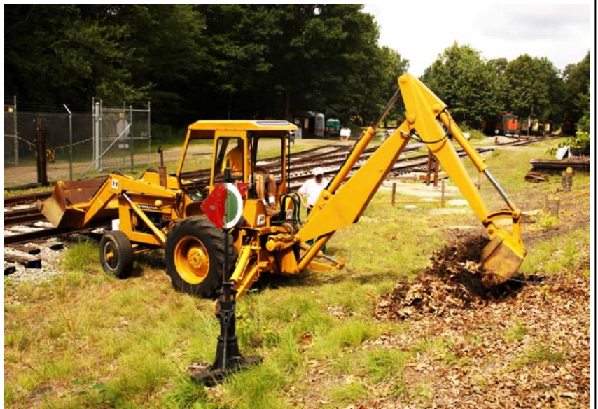
Dick Arnold operating his International Harvester backhoe is removing numerous stumps that need to be removed from the Gallows Signal Project site area. Just behind where the backhoe is operating is where the Gallows Signal will be constructed. (Robert A. LaMay Photo)
