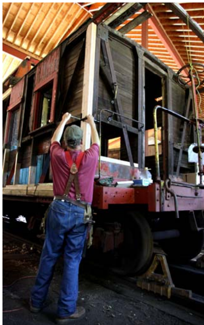
Duke York is installing a main corner support beam in the Central Vermont Center Cupola caboose no. 4052 inside the roundhouse. (Robert A. LaMay Photo)
