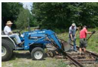
Trackwork is an on-going project as shown above. Ties are being replaced along certain sections along the eastern section of the Air Line. (Robert A. LaMay Photo)
