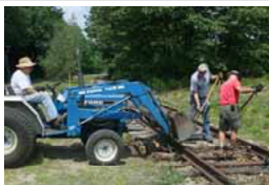
Trackwork is an on-going project as shown above. Ties are being replaced along certain sections along the eastern section of the Air Line. (Robert A. LaMay Photo)
