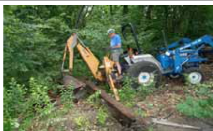
Bob Hassett is moving some old ties so they can be inventoried for future track work projects at the museum. (Robert A. LaMay Photo)
