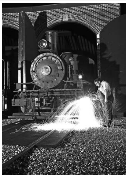
Rich Cizik does some metal work on Steam #10. Lights supplied by Steve Barry. (Robert A. LaMay Photo)
