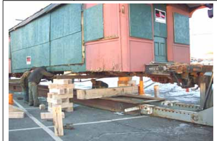
With both wheel sets (trucks) removed, the lowering begins. Note the trailer underneath the car. Plan is to lower the car onto this trailer, connect the wheels and harness assemblies, and off it goes.
