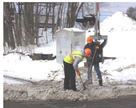
New England Central RR crews chip ice away from Bridge St. crossing. Note snow pile in background. (Robert A. LaMay Photo)
