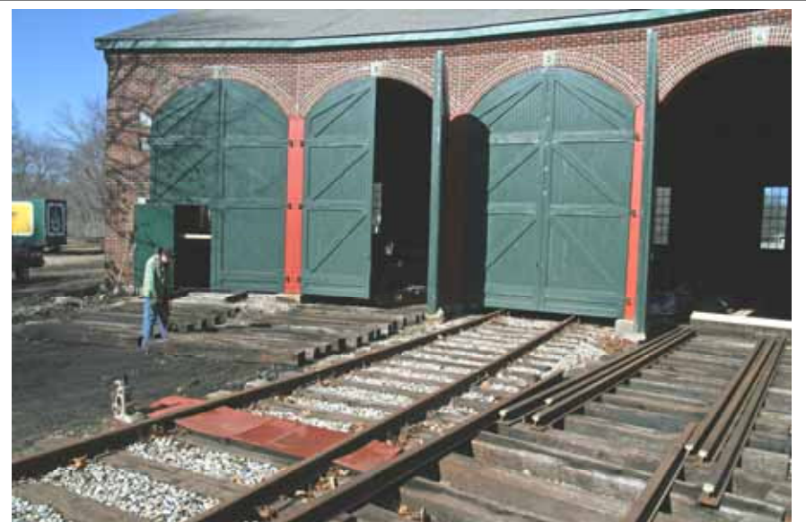
This 02/28/09 photo shows member Rolf Johnson moving ties into position in front of pits 1 and 2. (Robert A. LaMay Photo)
