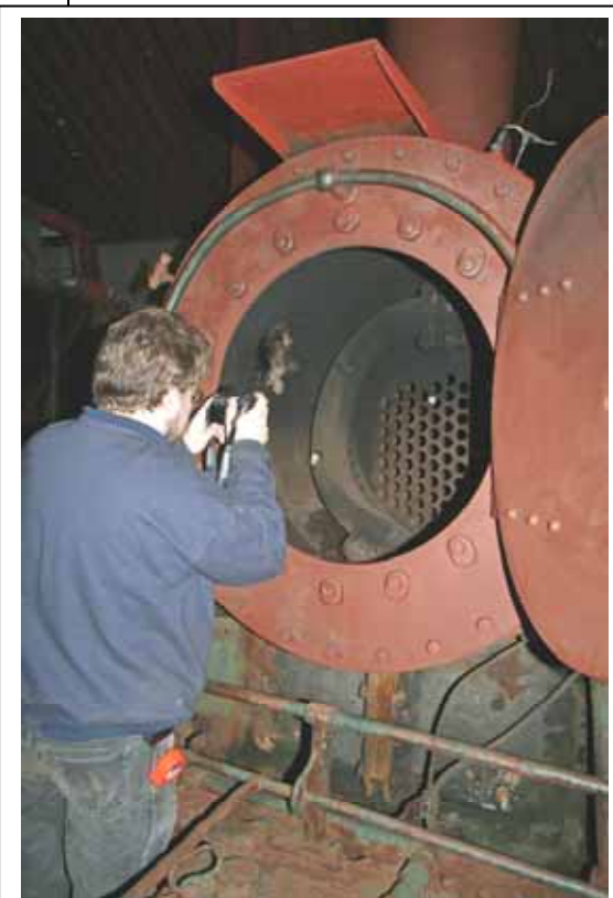
Jamie Key takes photos inside the boiler of Steam No. 10 for a mapping project. (Robert A. LaMay Photo)
