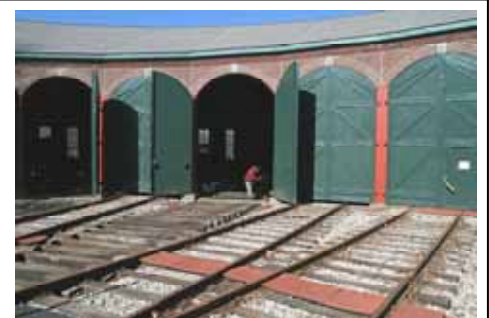
This photo taken 02/21/09 shows the track configuration of pit tracks 3 to 6. (Robert A. LaMay Photo)
