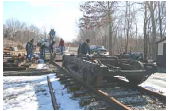
This shows the second wheel set after it was unloaded and the hook is about to be taken off. (Robert A. LaMay Photo)
