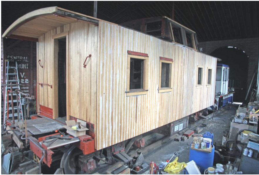
This photo taken 12/11/12 shows the finished wood section of the Central Vermont Center Cupola Caboose number 4052 car-body. Interior work will continue as will the metal work on both ends. (Robert A. LaMay Photo)
