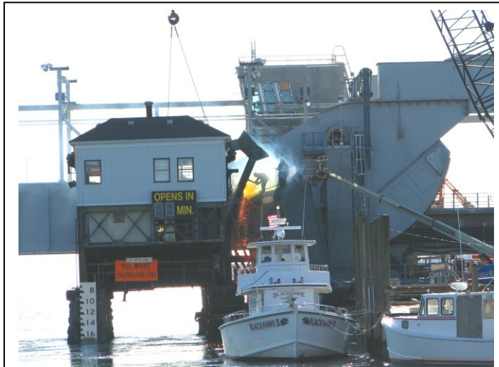
This photo shows workers in center of photo taking bridge apart at Niantic, CT. Taken 11/9/12 by resident Anne Wilcox.
