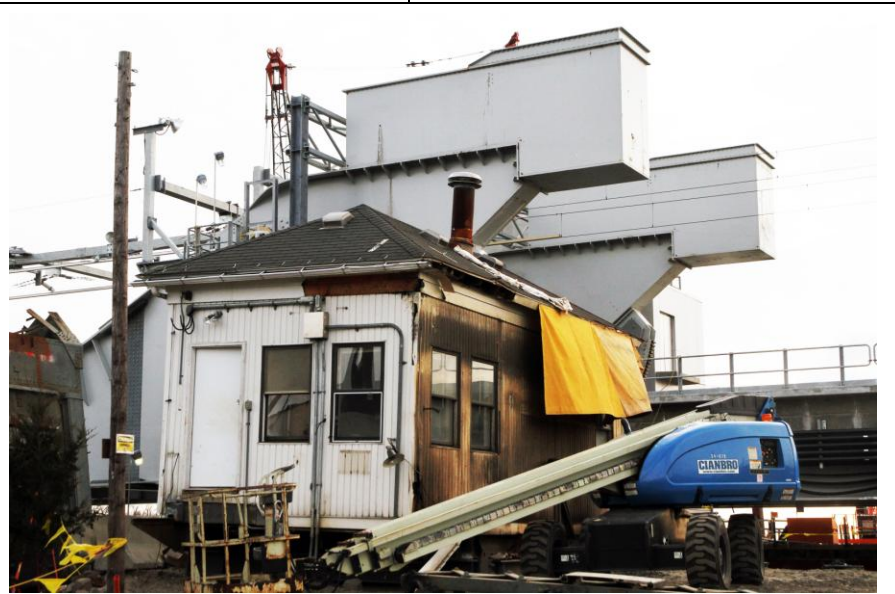
This photo taken 11/25/2012 shows the Niantic Draw-bridge shanty sitting on the ground next to the new bridge. The next step is having it transported to the Connecticut Eastern Railroad Museum located in Willimantic, CT. (Taken with permission by Robert A. LaMay)
