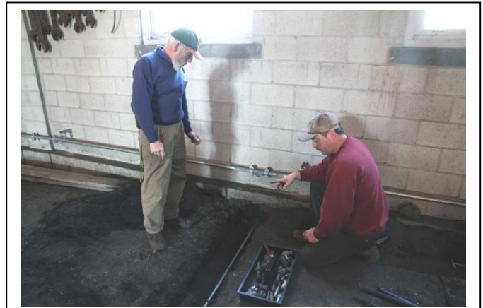
Bob Hassett on left and Bill Voorvaart discuss the compressed air lines that are being installed in each of the six inspections pits and other areas inside the roundhouse. (R.A. LaMay Photo)
