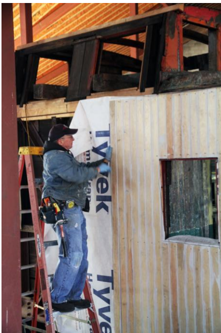
William Bouchelle applies new pieces of wood to the Central Vermont Caboose number 4052. (Robert A. LaMay Photo)
