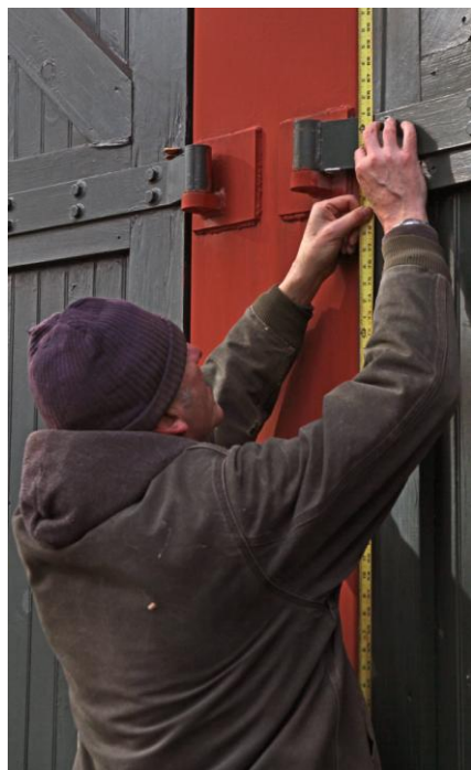
Art Hall, Jr. measures the metal strap on Pit number 2 round-house doors. The museum is designing a lighter, stronger and more durable door. (Robert A. LaMay Photo)
