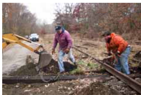
Rolf Johnson and Rich Cizik, Jr. help with the installation of a replacement tie. (Jean Lambert Photo)
