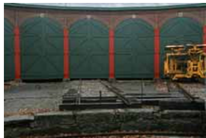
This photo shows the latest progress on pit track No. 3. (Robert A. LaMay Photo)
