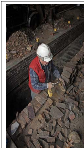
Adrian Atkins inspects each brick to make sure it is clean will make a proper fit in Pit #2. (Robert A. LaMay Photo)
