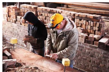
Bill Voorvaart (R) along with his son Tucker are making brick dust which will be used along with sand to form a bed on which the brick floor will be placed in the bottom of Pit number 2. (Robert A. LaMay Photo)
