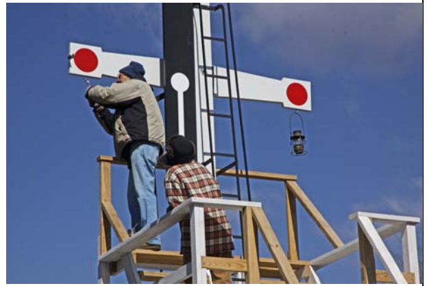
Dick Arnold installs lantern hangers as Carol Stanich looks on. (Robert A. LaMay Photo)
