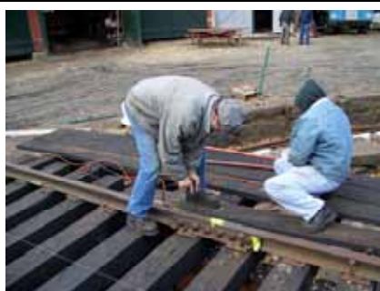
Mark Granville and Bill Bouchelle work on tying rail down to turntable bridge. (Andy Fischer Photo)
