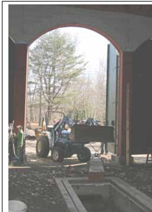
Bob Hassett with 'Big Blue' moves timber into Pit No. 4 for eventual placement. (Robert A. LaMay Photo)
