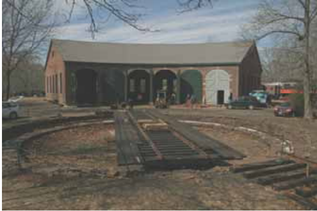
Photo taken March 22 nd shows the latest progress with rail on the turntable bridge. Rail from the turntable to the roundhouse should begin soon. (Robert A. LaMay Photo)
