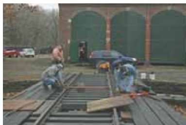
Jeff Laverty, Mark Granville, and Bill Bouchelle continue to align the rails on the turntable bridge. (Robert A. LaMay Photo)
