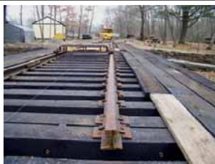
Here is an unusual view of the finished rail on the turntable bridge. (Andy Fischer Photo)
