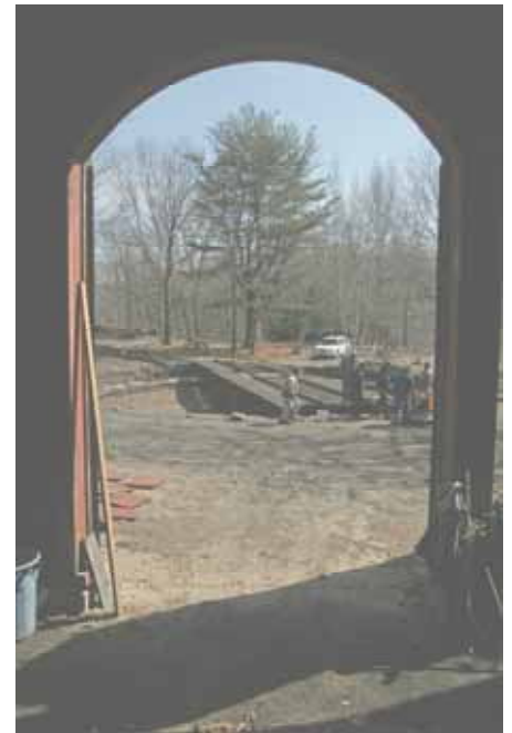
This view from inside the roundhouse shows the rail on the turntable bridge. Soon we will be able to see equipment move in and out of the roundhouse. Come see June 8 th at 1:30PM. (Robert A. LaMay Photo)
